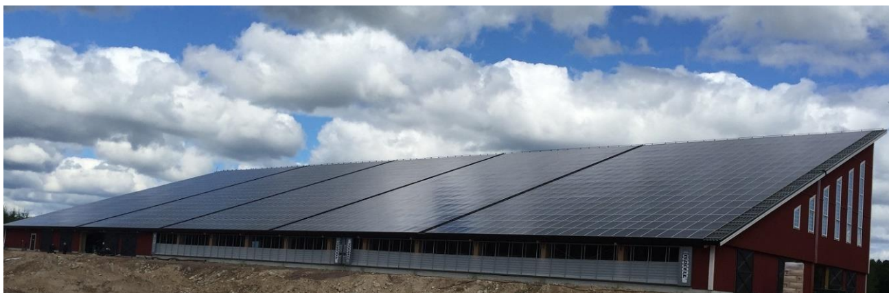
Picture of the solar PV installation at Nöbble Solpark in Kalmar. Photo credits ©: Kalmarsund Vind
